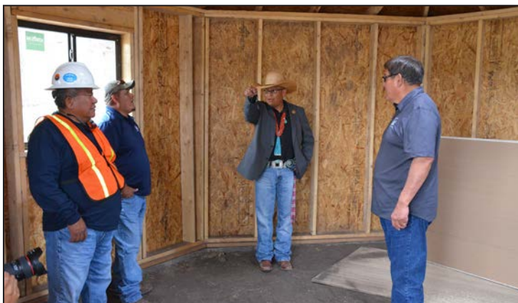
PHOTO: Speaker LoRenzo Bates and Council Delegate Steven Begay visit a hogan under construction in Naschitti, N.M. on Aug. 21, 2018.
